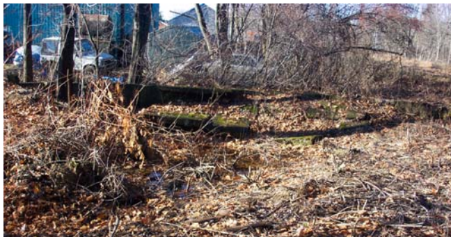
Figure 13. Debris covering turntable pit foundation, (HWA, 2004).
