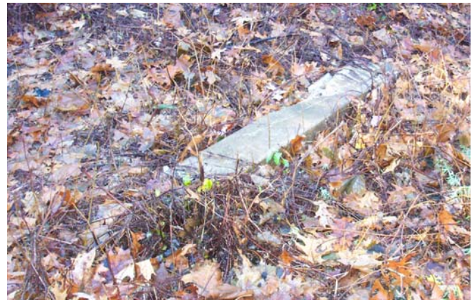
Figure 12. Toppled and broken whistle post, (HWA, 2004).
